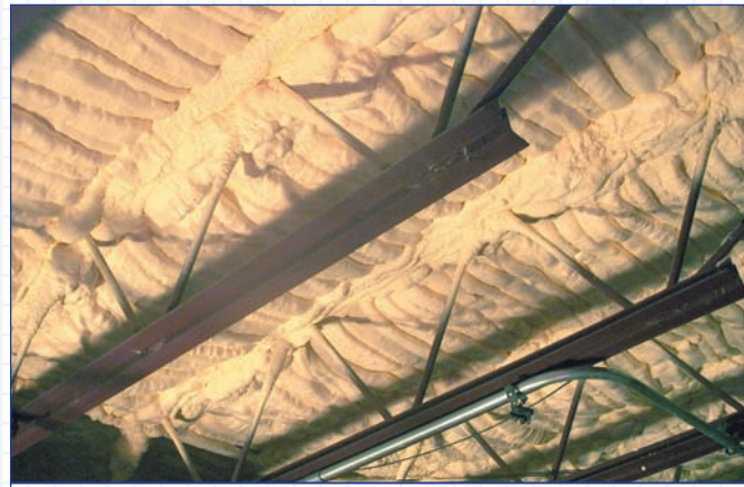
Area of application for Icynene® included the footprint of the chillers and walk-in freezers plus a perimeter area extending 10 feet beyond.
