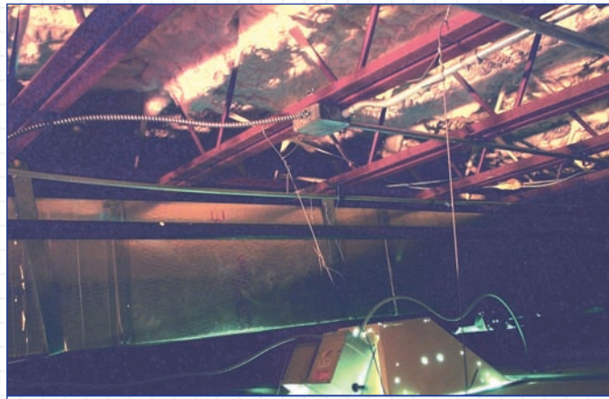
Icynene® insulation applied directly to the metal ceiling area below the chillers and walk-in freezers.
