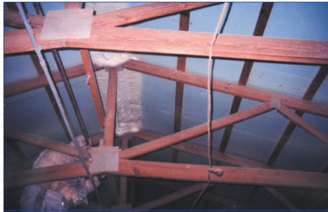
Sealing of the ridge vent with Icynene® Insulation to prevent air leakage.
