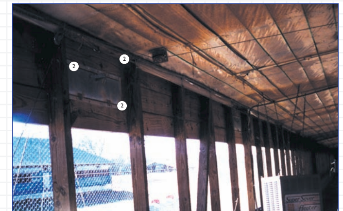
(2) The gaps between these boards allowed substantial air leakage.
